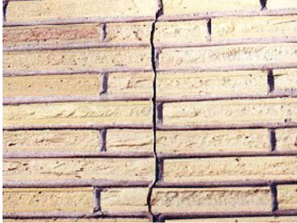
Fireplace air leakage
